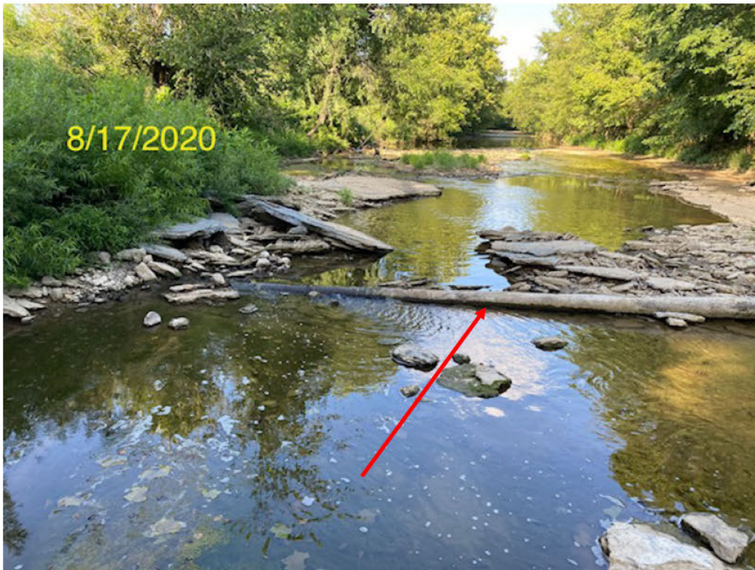
Figure 9. Photo of 77-year old LG & E Calvary Natural Gas Pipeline exposed across Cox's Creek channel. The Calvary Natural Gas Pipeline is often impacted by logs, debris and rocks during flooding and by off-highway vehicles during low flow. Photo by Kim Rummage.
