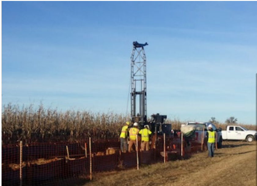
Figure 13. Photo of LG & E contractors drilling bore holes for some secret purpose; several were drilled to depths of 340'. LG & E conducted drilling in violation of permit applications and may have damaged aquifers and ground water sources used for drinking water.
